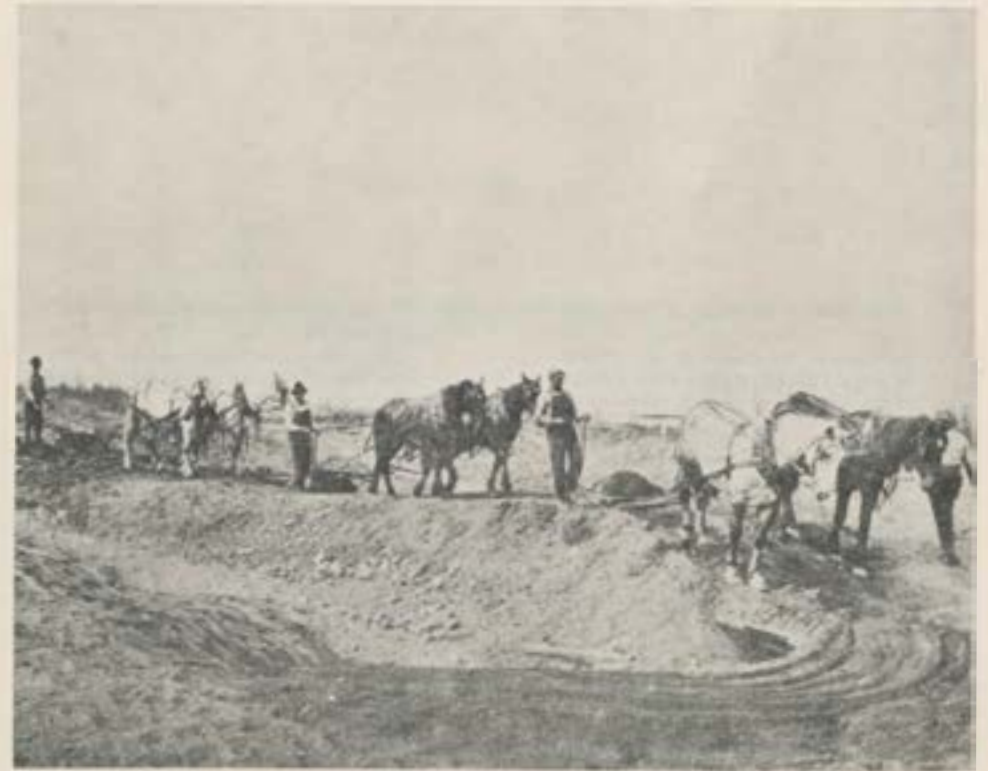
Building roads with drag scrapers and teams during World War I period
